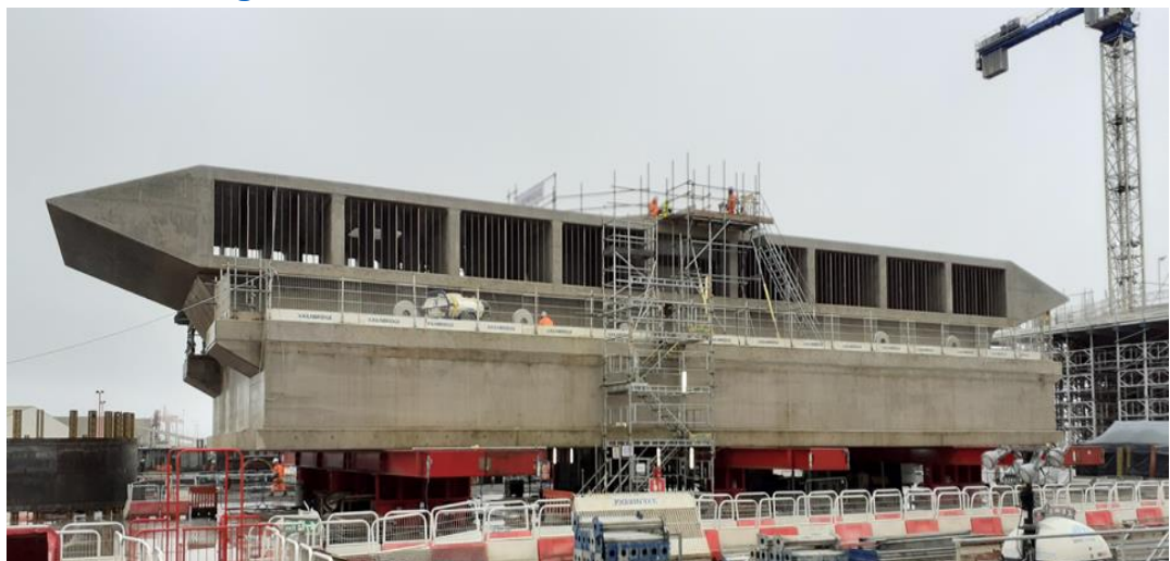
Figure 6.4: one of the Hinkley Point C intake heads being constructed. A similar design will be installed at Sizewell C.
