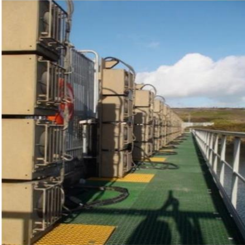
Figure 7.1: Sound projector units at Pembroke CCGT
